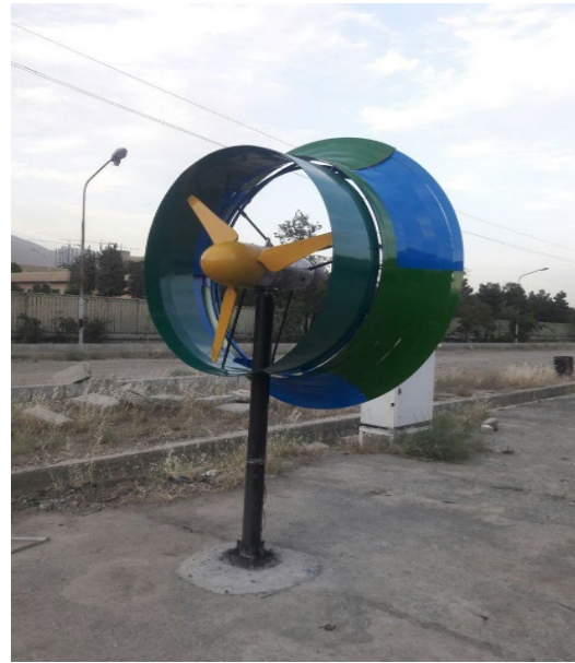
Figure 7. Installed TMWT in agriculture department of TMU.
