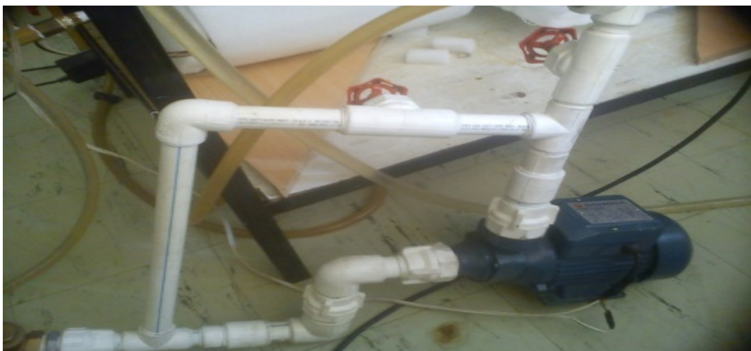
Figure 3. A view of centrifugal pump.
