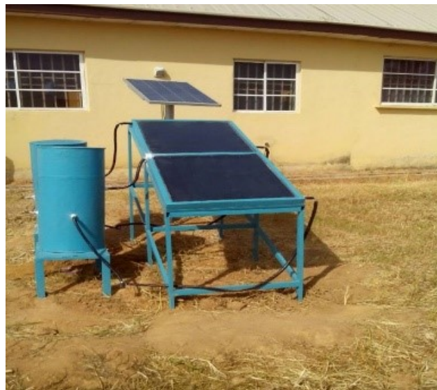
Figure 6. The developed and installed solar heating experimental setup
