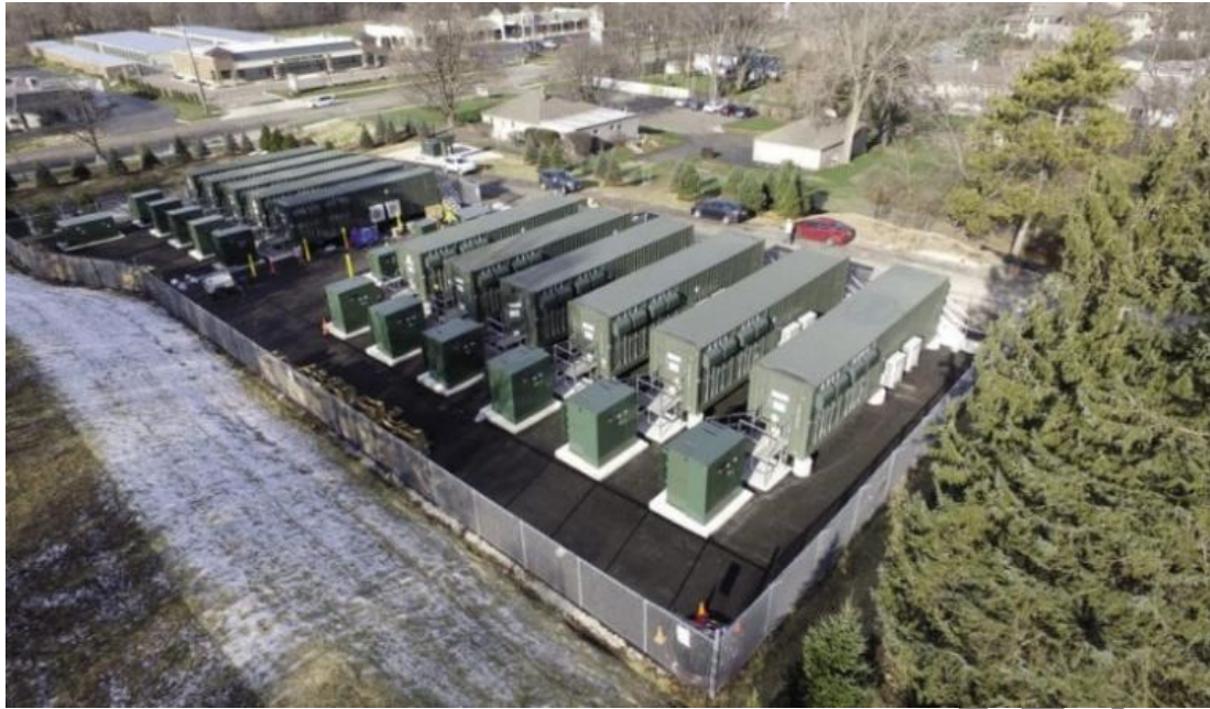
Figure 8. BESS located near load center
