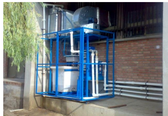
Figure 6. Photograph of the solar LDAC absorber unit as viewed on the site
