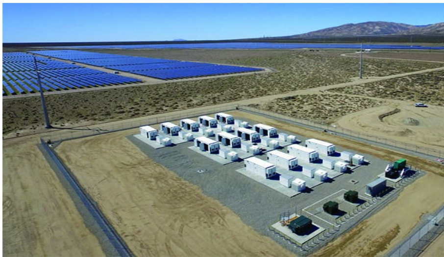
Figure 9. BESS co-located with PV plant
