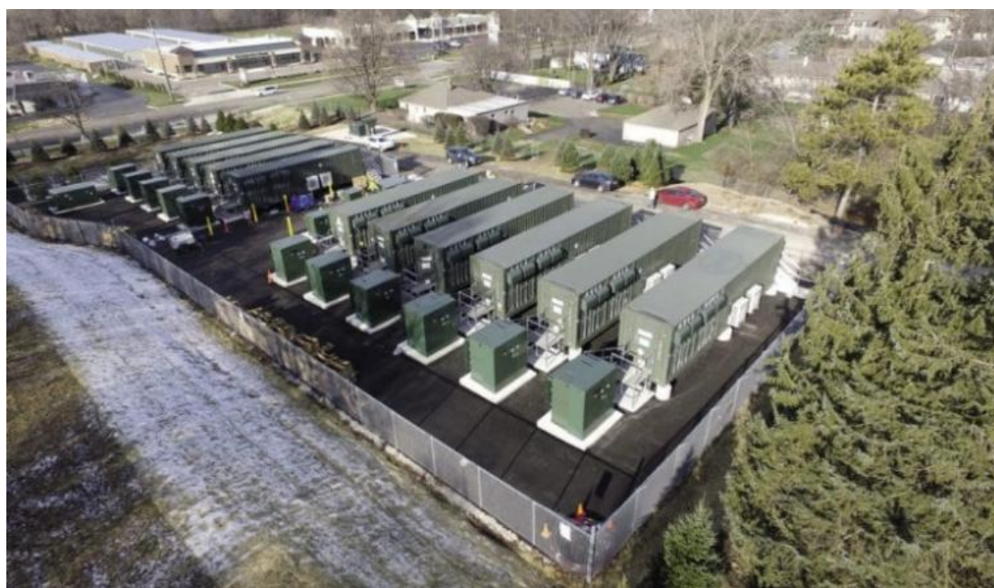
Figure 8. BESS located near load center
