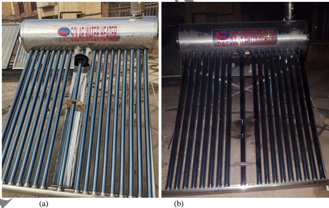
Figure 5. (a) ETSC after installing the parabolic concentrator; (b) experiment setup without the concentrator
